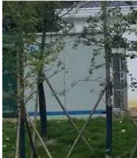
On-site installation picture
